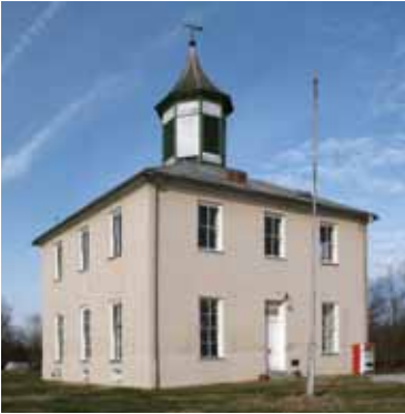
A low-interest loan from Indiana Landmarks allowed the Rome Community Center to repair a leaking cupola atop the 1819 old Perry County Courthouse.
