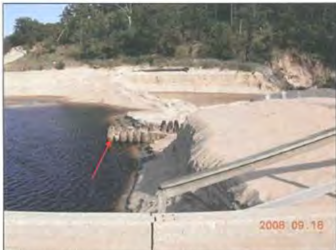
Photograph 3: Historic posts revealed as a result of erosion from flooding (Note – this photograph was taken prior to filling/stabilization of the washout. These elements are not currently exposed.)
