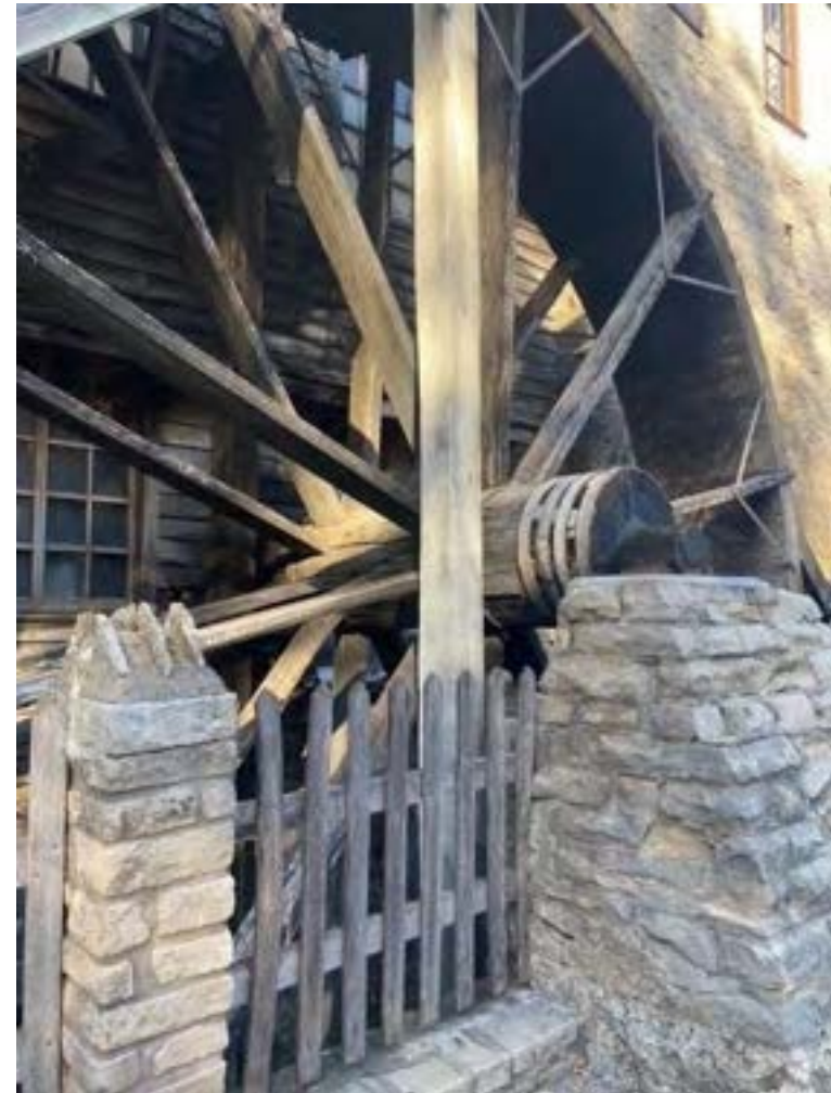
Wheel and shaft to be replaced
