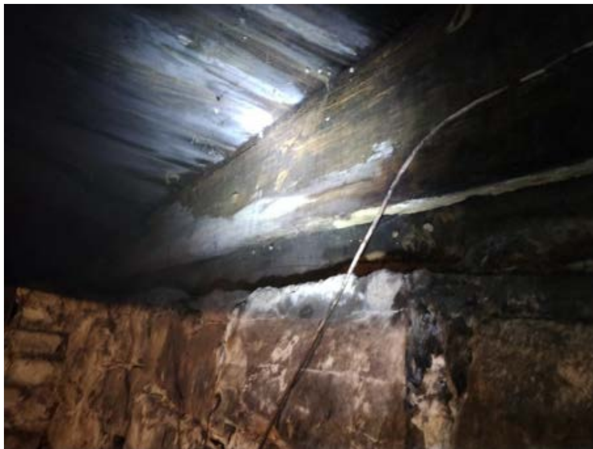
View from basement of damaged sill
