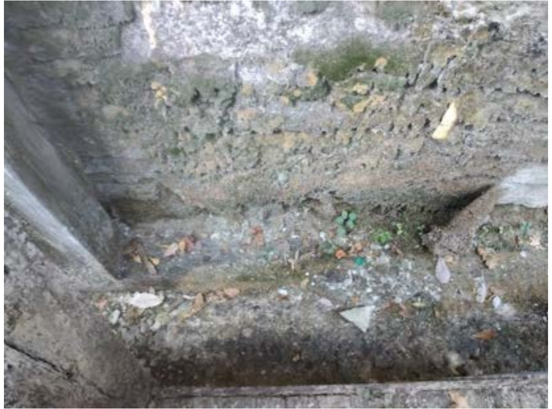
Lichen on stone needing cleaned to inspect mortar
