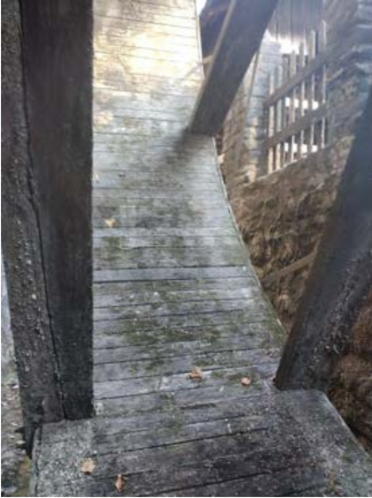
Standing inside the wheel view of rotting wood
